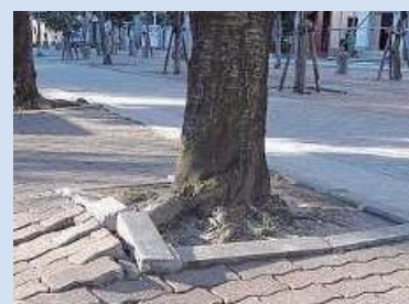
Uneven sidewalks due to roots rising out of the ground
