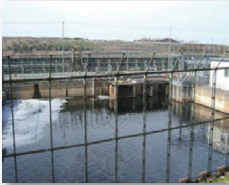
Receiving Reservoir (Pump well)
