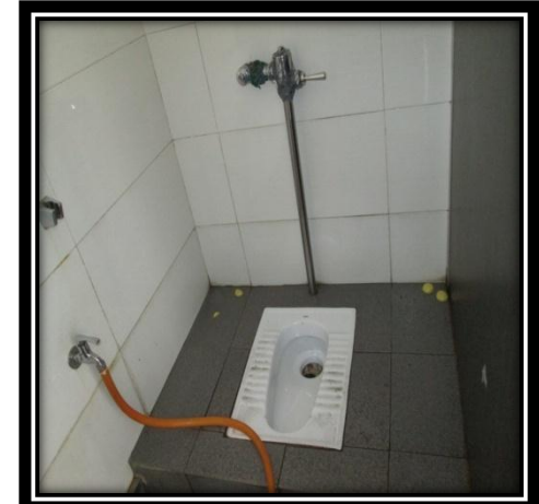
HOSE ON THE FLOOR
