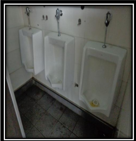
WET AND DIRTY URINAL
