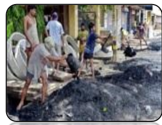
Silt Generated from drains upto 4ft. 31 January 2015
