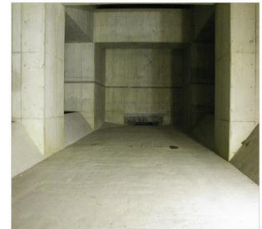
▲ Minamisuna rainwater reservoir for flood control The upper part is used effectively as collective housing etc. (the amount of storage of 25,000 m 3 ).
