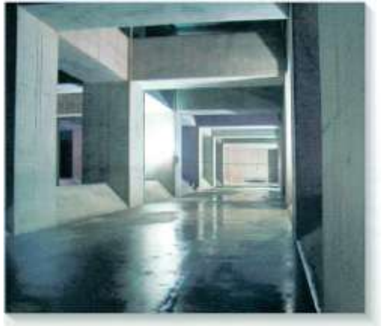
Stormwater regulating reservoir
