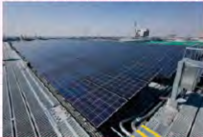
Solar power generation (2-1 Marunouchi precinct)
