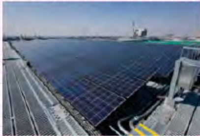
Solar power generation (2-1 Marunouchi precinct)
