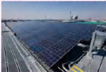
Solar power generation (2-1 Marunouchi precinct)
