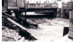
Taishido, City of Setagaya: Condition of collapsed revetments near Karasuyama River's Taishi Bridge
