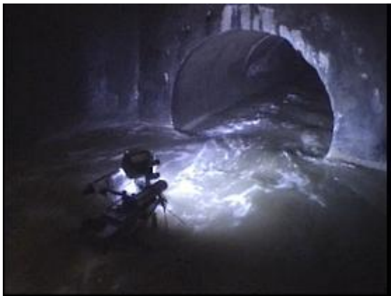
Camera system for examining large-caliber pipe (conduit)
