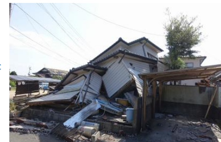
A wooden house built to the pre-2000 standards that collapsed due to the Kumamoto earthquake
